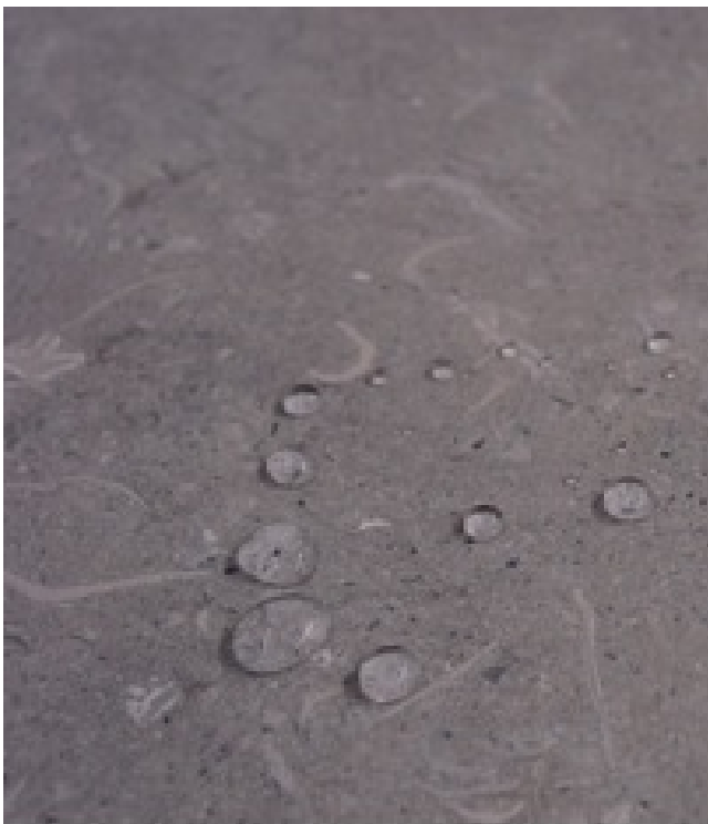
Fig 1 . Before the removal of invisible sealer residue, shows high water beading.
