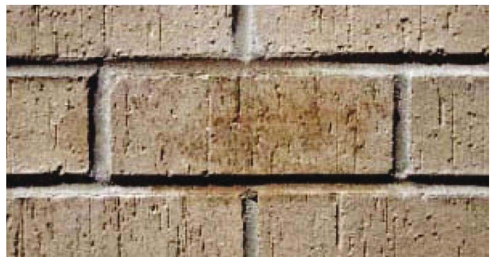
Manganese deposit on brick and grout joint
