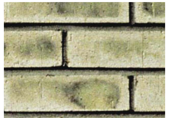
Vanadium sometimes incorrectly identified as mildew or bacteria
