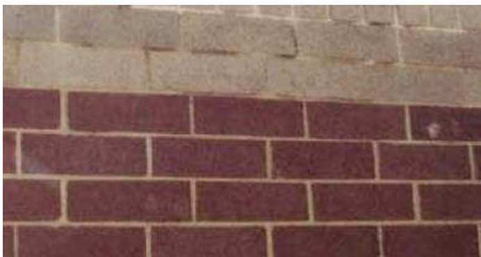
Manganese staining in the grout joint
